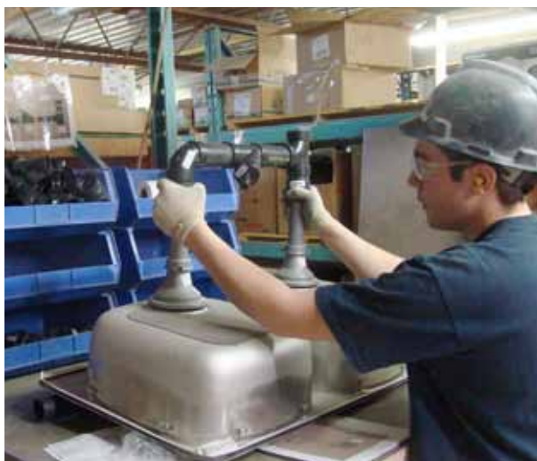
Nathan Titus preassembles a sink unit, so the plumber can focus on connecting the sink to the new home.
