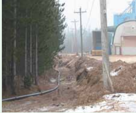
The pipeline from Embers to NSS&G
